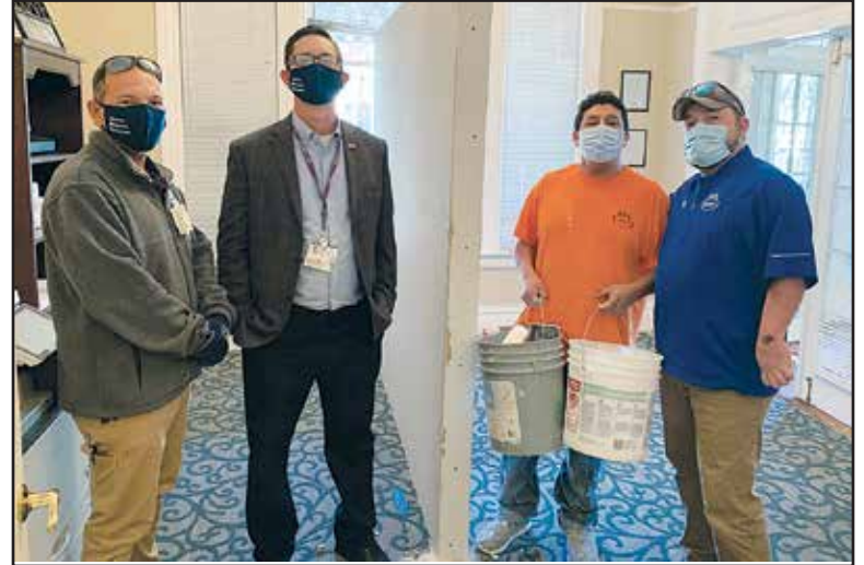
Medexcel Lead Mechanic, Cosmo Trinca, observes as supervisor Kevin Darnel reviews plans for the new business cubicles with CCS workers Brian and Ramos • CCS donated the construction of the wall and the cubicles • Medexcel provided the butcher block desk top
